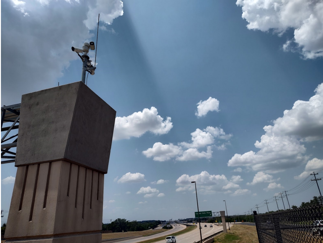
Closed Circuit Television (CCTV)
