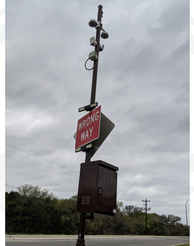
Wrong Way Vehicle Detection System (WWVDS)
